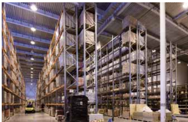
High bay lighting
